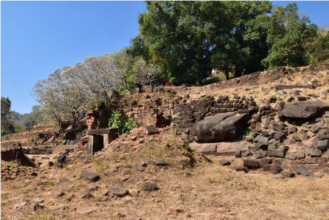
Fallen structures of 3 rd terrace
